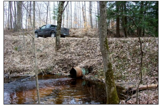
Haze Road crossing on a tributary to the Betsie River impedes fish passage. The crossing will be replaced by a large elliptical culvert, allowing natural flow and upstream fish passage..
